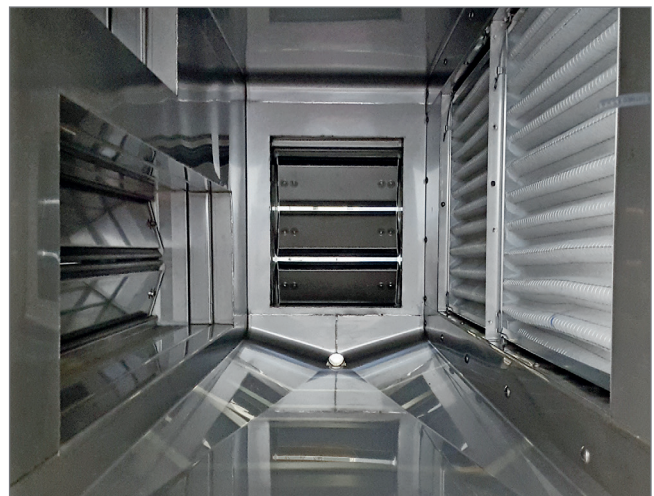
SLOPED DRAIN PANS
